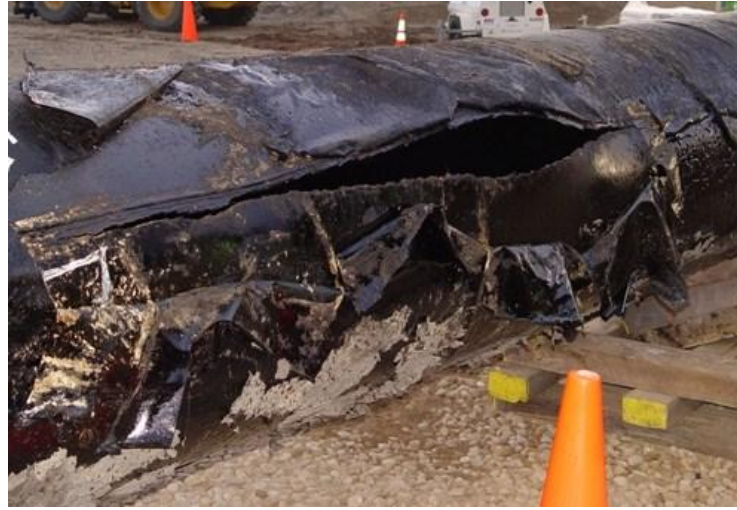
Figure 1: Example of the through crack in a fractured pipeline
